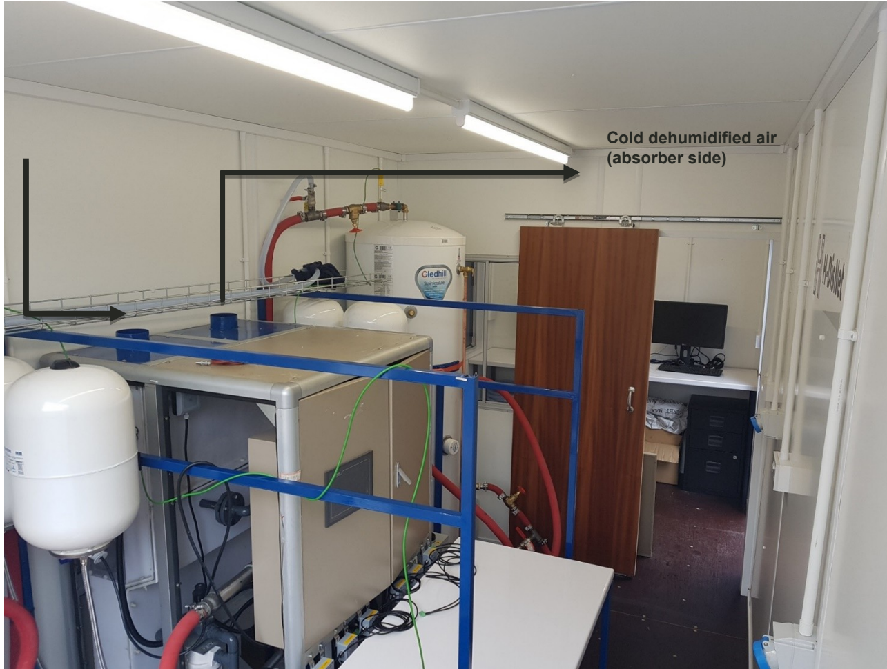
Thermally driven liquid desiccant fresh air system
