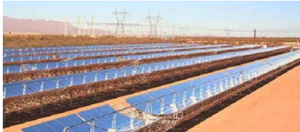
CSP Solar Plant
