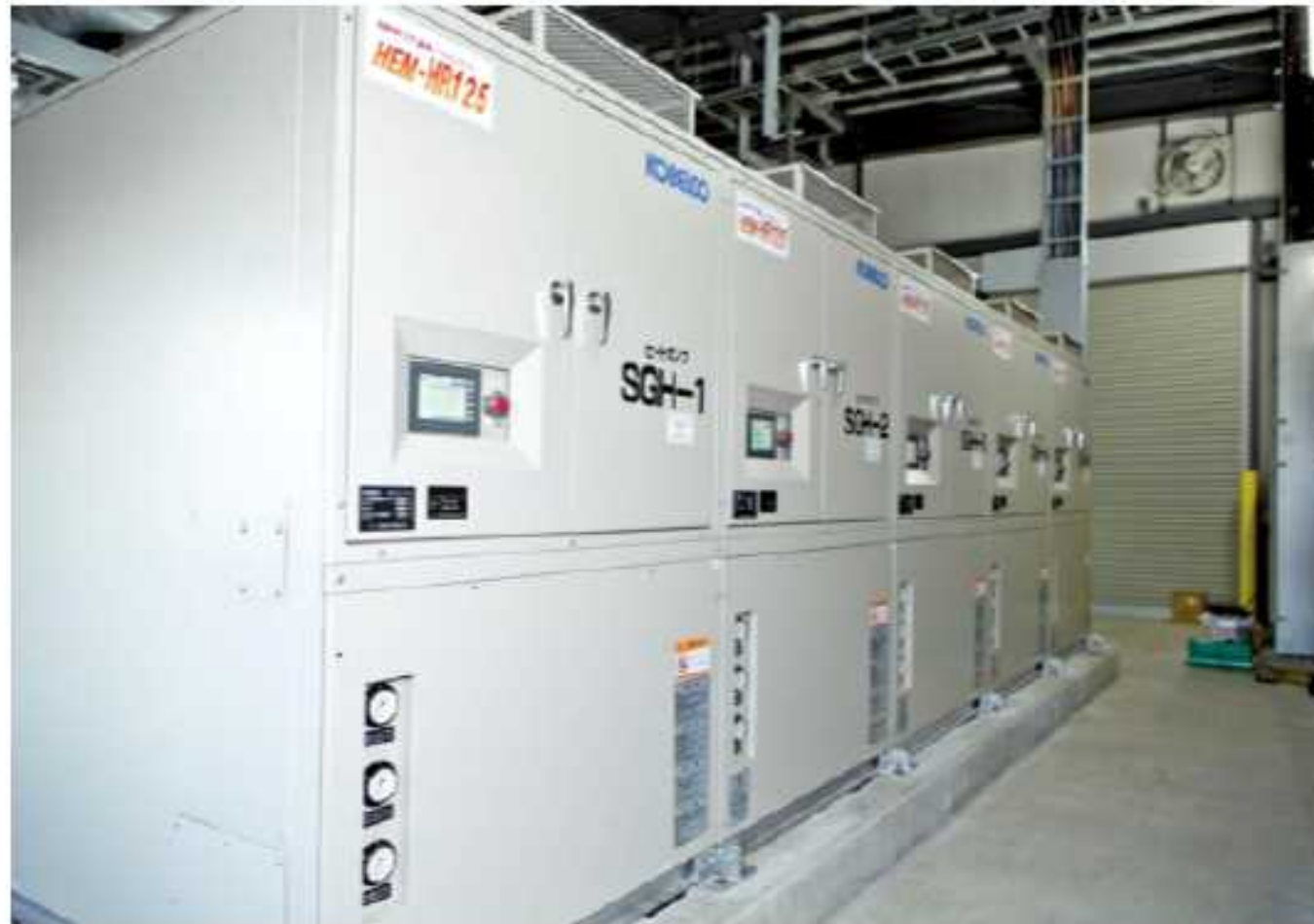
Figure 1: Steam supply heat pumps
