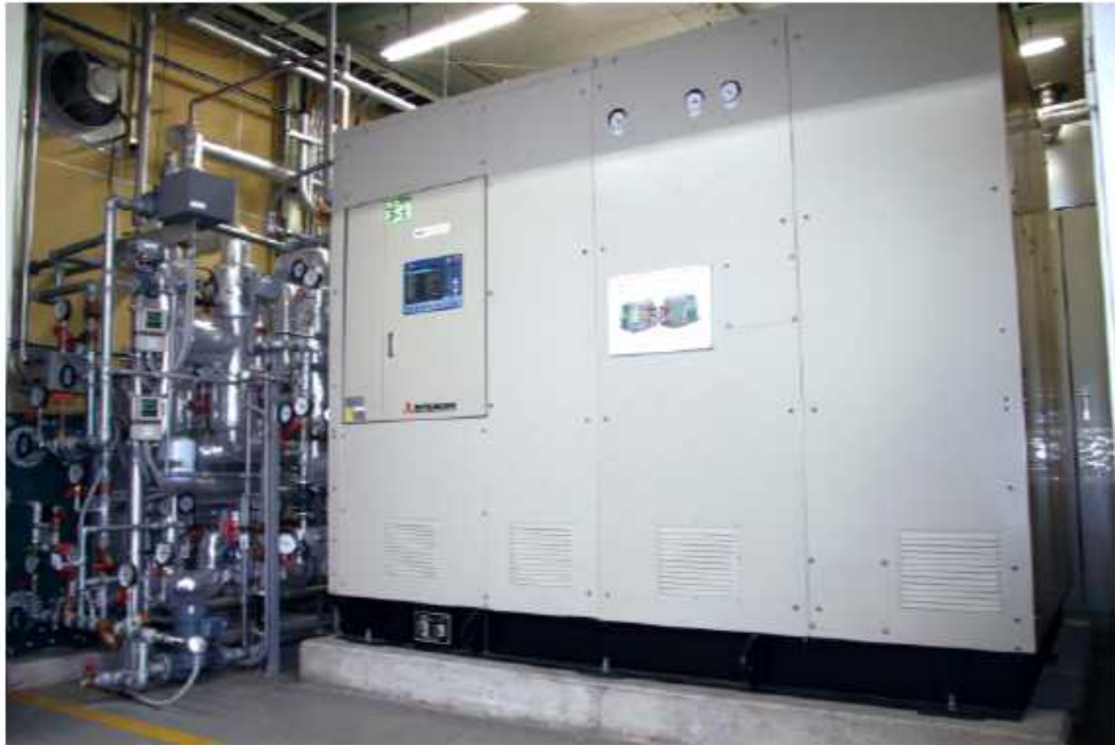
Figure 1: Hot water supply heat pump
